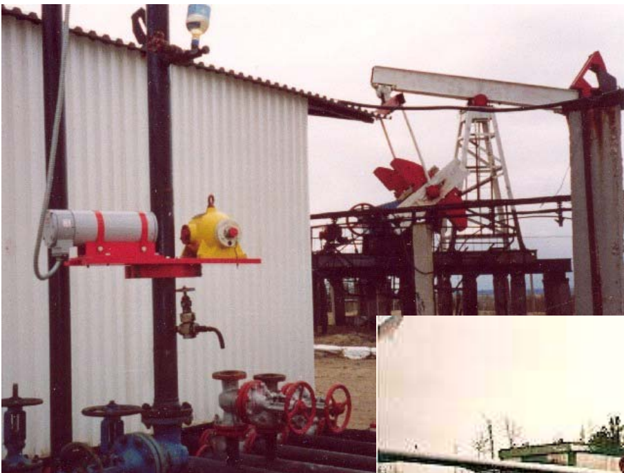
Single meter on beam-pump well
