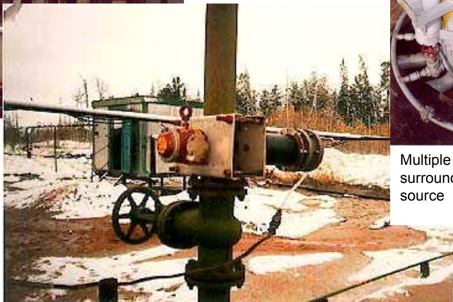
Prototype in field installation
